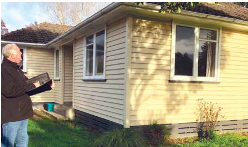
This Kummer Crescent property is about to undergo a refurbishment to bring it into line with the Healthy Homes Standards.
